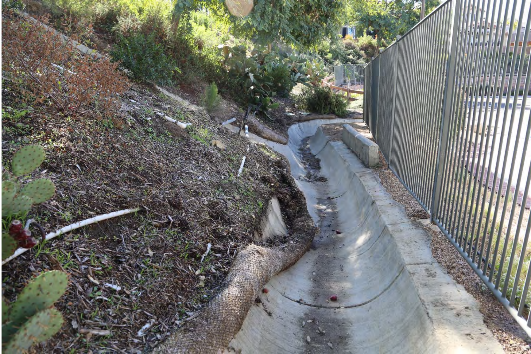
Dead plants, erosion, straw wattle falling along the entire length of the swale
