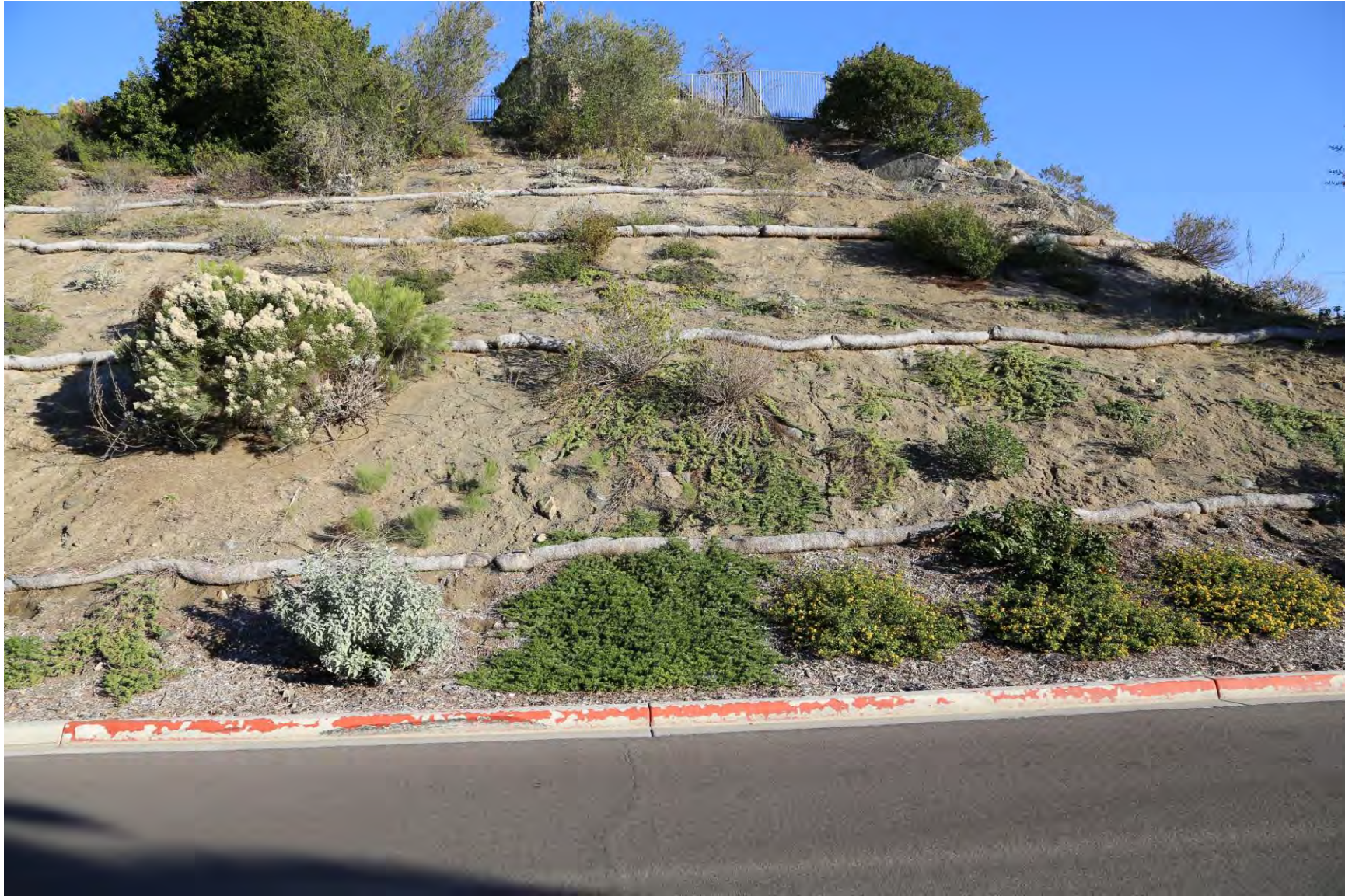
Exposed ground, erosion
