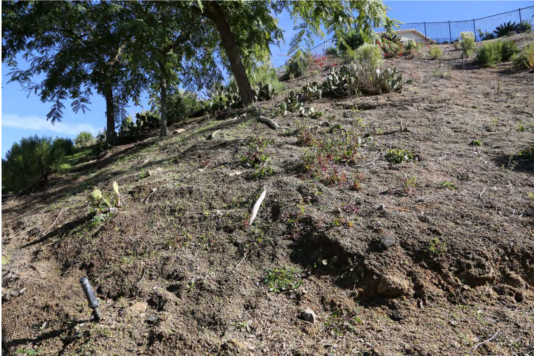
Exposed ground, erosion, failed hydroseed (gap in irrigation at the top), tree roots exposed
