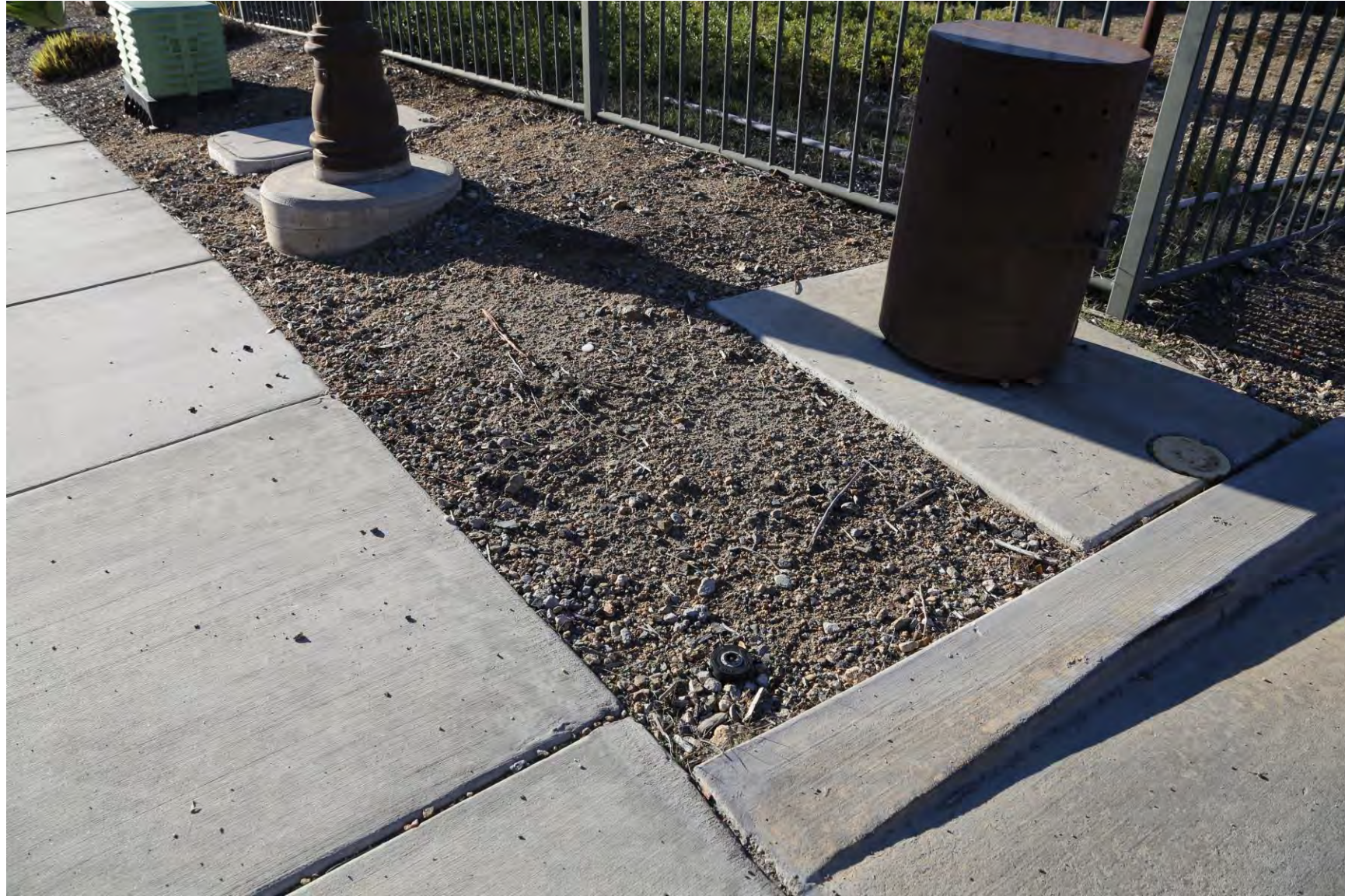
Exposed ground, sprinkler to nowhere, shrub gone
