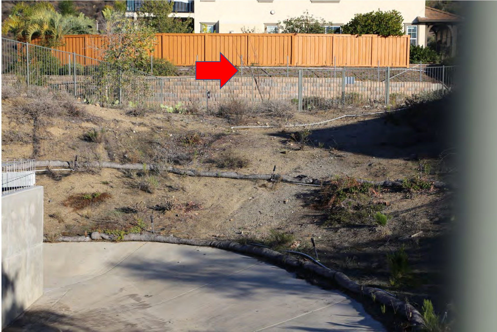
Dead tree, exposed ground, erosion
