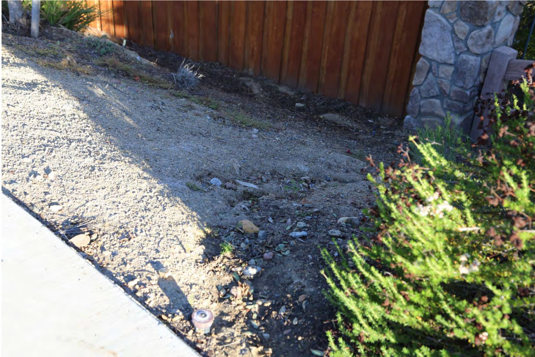
Sprinkler obstructed, ground erodes over the bottom of homeowner fence
